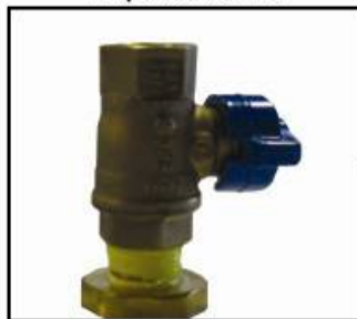
Manual Shut-Off Valve for Propane Supply Installed in Propane Inlet Port
